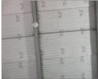
Photo of fire safety equipment Smoke detector.JPG
