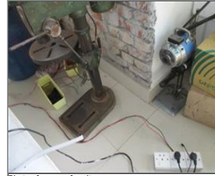
Photo of non-conformity Loose connection in maintenance room.JPG
