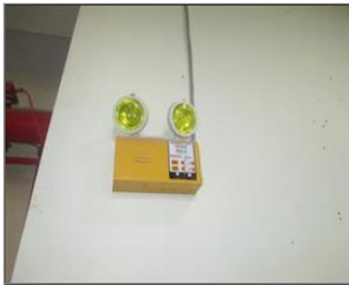
Photo of fire safety equipment Fog light.JPG
