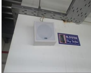
Photo of fire safety equipment PA system.JPG
