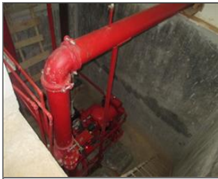
Photo of fire safety equipment Fire pump.JPG
