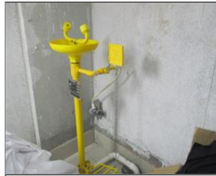
Photo of the inside of the main production hall Eye wash station.JPG
