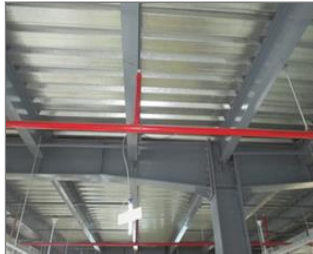
Photo of fire safety equipment Sprinkler system.JPG
