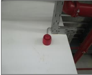
Photo of fire safety equipment Fire Alarm.JPG
