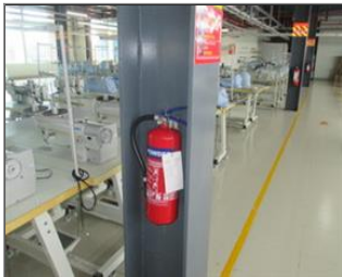
Photo of fire safety equipment Fire extinguisher.JPG
