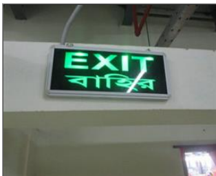
Photo of fire safety equipment Exit light box.JPG
