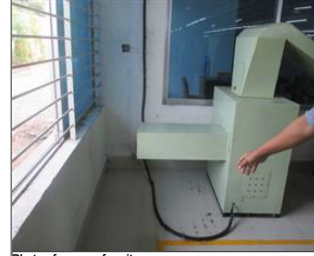
Photo of non-conformity Ducting system missing for thread sucker machine.JPG
