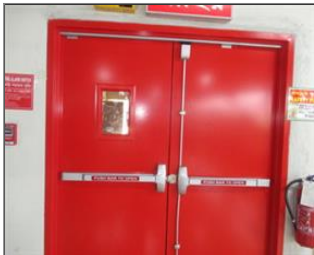
Photo of fire safety equipment Fire door.JPG
